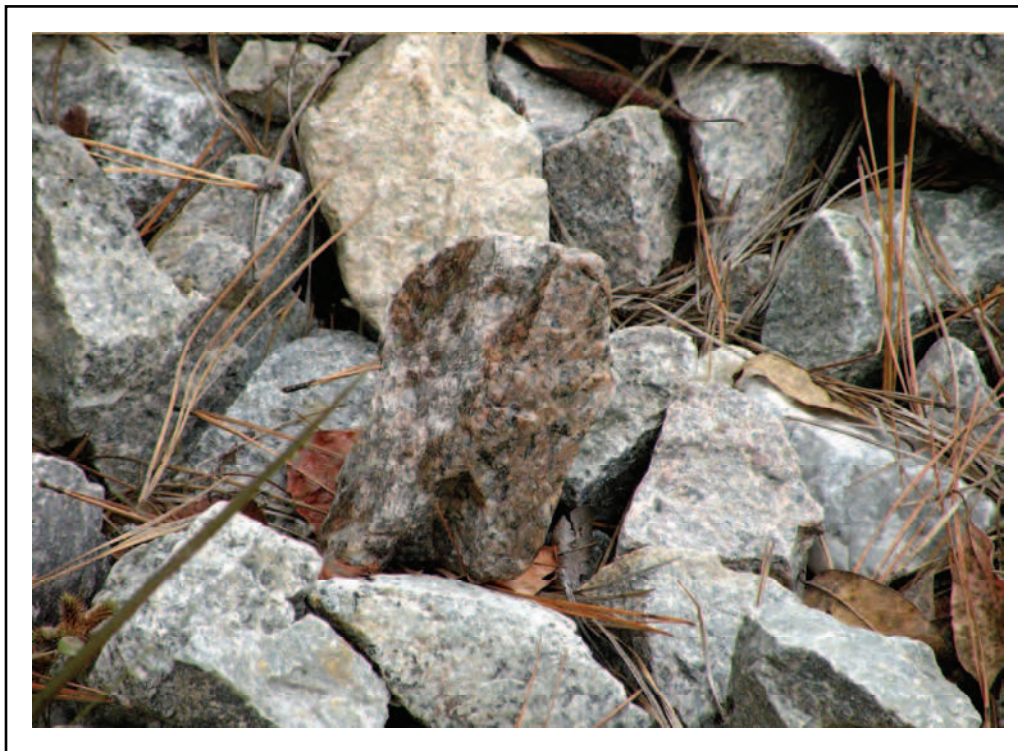
Figure 1-27. Staining at creek (center rock is wet while the remainder of the rocks are dry)
